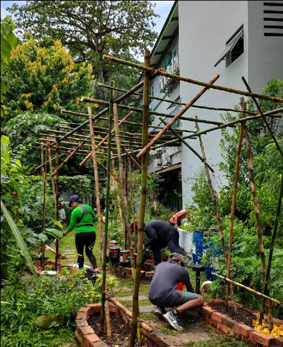
CONSTRUCTION OF A BAMBOO PERGOLA AT THE MAKE A DIFFERENCE FAMILY GARDEN
