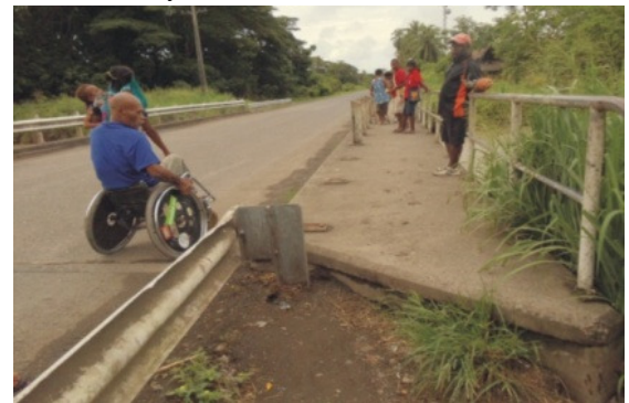
Photo: A wheelchair user attempts to access a bridge footpath constructed without ramps.
