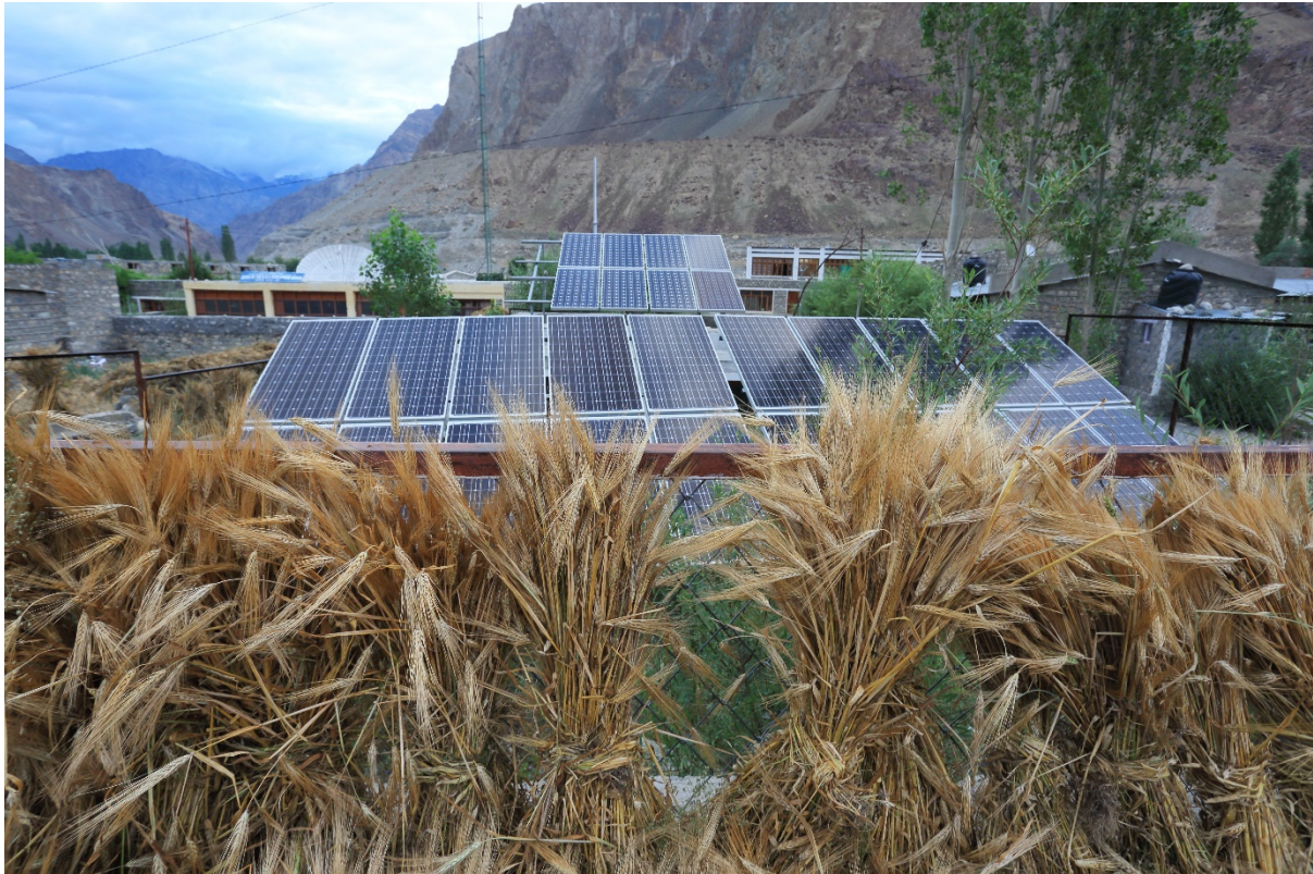
Figure 8.5 Solar panels in Turtuk village north India
